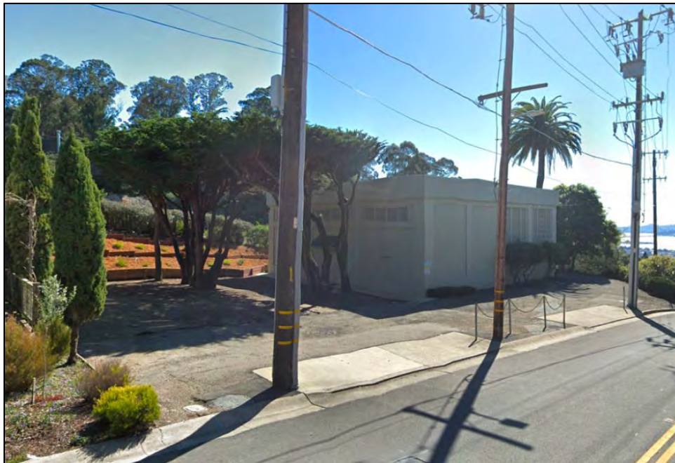
Figure 17: PG&E Substation (Source: Alternatives Analysis).
